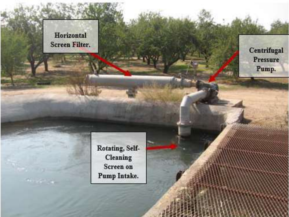
Figure 6-7 Rotating, Self-Cleaning Screen Filter Followed by Centrifugal Pressure Pump and Horizontal Screen Filter for Almond Irrigation
