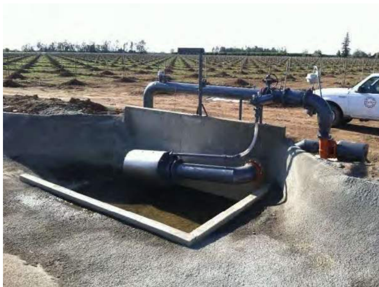
Figure 3. Alternative turnout structure to allow direct pumping from district canal to supply an on-farm pressurized irrigation system. During and following construction.
