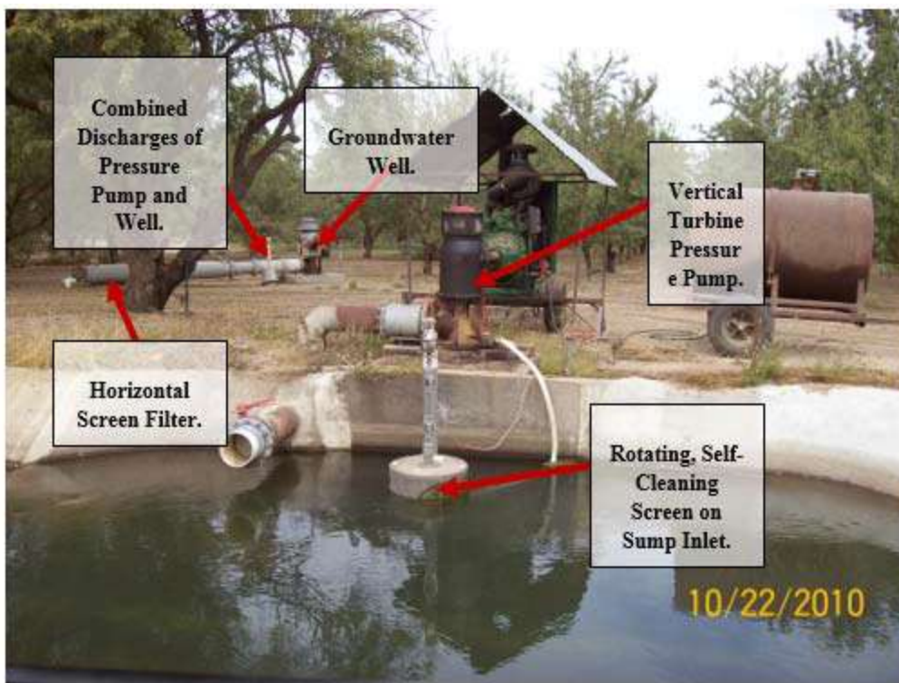
Figure 6-9 Rotating, Self-Cleaning Screen Filter Followed by Vertical Turbine Pressure Pump and Horizontal Screen Filter for Almond Irrigation. Screen Filter Installed Downstream of Combined Discharges of Pressure Pump and Groundwater Well
